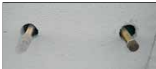
Figure 3.3.2 Neat finishes of installed services
