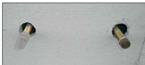
Figure 2.6.2 Neat finishes of installed services
