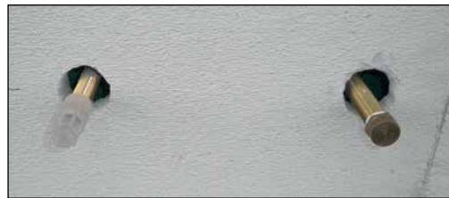
Figure 3.3.2 Neat finishes of installed services
